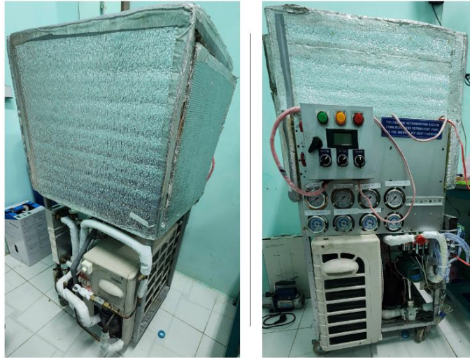
Figure 2. Photos of R513A/R744 cascade system
